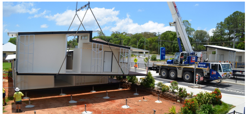
■ New Junior School Office administration block being placed in to position during the holidays. More pictures of all development projects can be viewed online at www.facebook.com/RedeemerLutheranCollege
